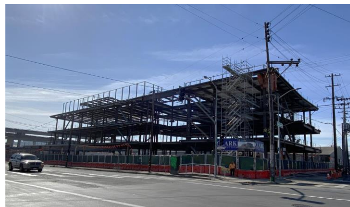
North and West Elevations – View from Intersection of Evans Ave. & Toland St. (February 27, 2020)
