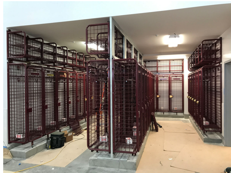
Firefighters' Lockers in Apparatus Bay (February 27, 2019)
