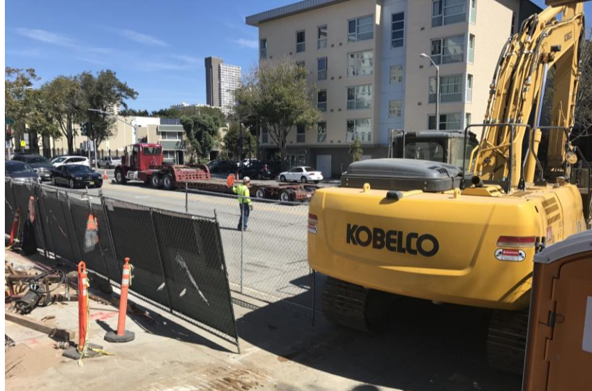
Watch for flaggers when large equipment enters and exits the project site (September 19, 2017)
