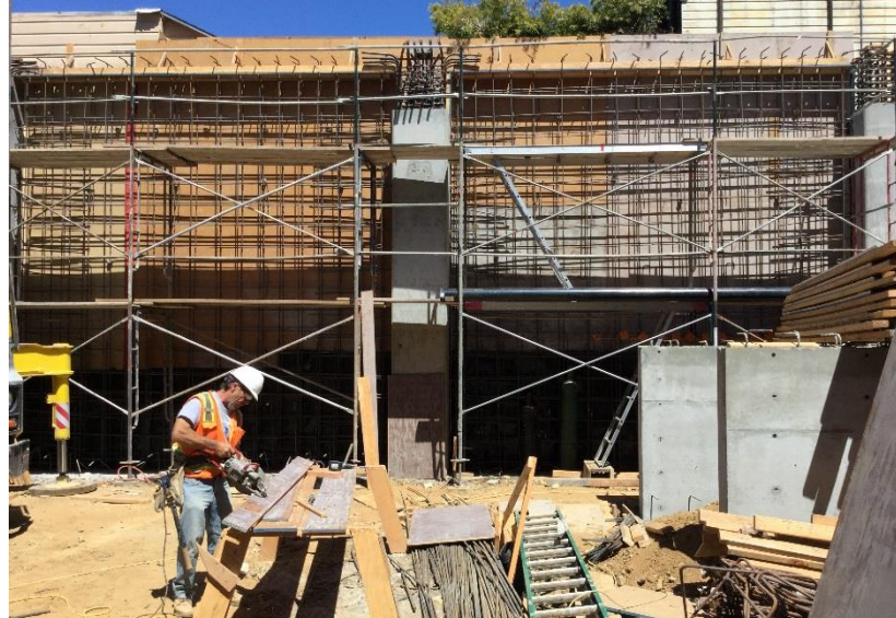
Building temporary scaffolding for access to East and West walls during shotcrete work scheduled for 7/24 and 7/25.
