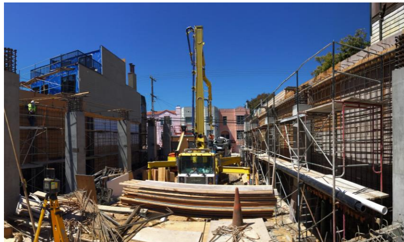
Pouring concrete for the grade beams at the 1st floor upper level (July 20, 2017).
