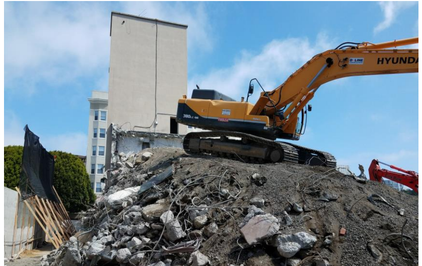
Materials compacted for access to the tower; barrier installed at West elevation to protect neighboring property from debris (June 5, 2017)
