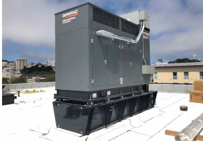
Emergency Generator Set at Main Roof (August 1, 2018)
