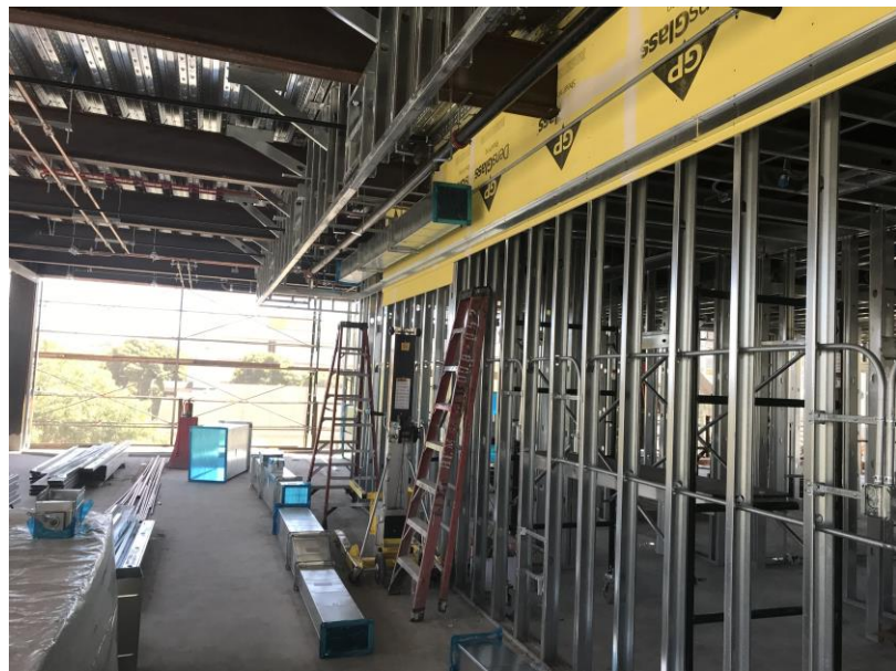
Metal Stud Framing and MEP Rough-In at Dormitory on 3rd Floor (May 9, 2018)
