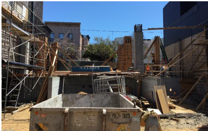
Formwork and rebar installed at 1st floor upper level columns and scheduled to be poured in Thursday 8/3.
